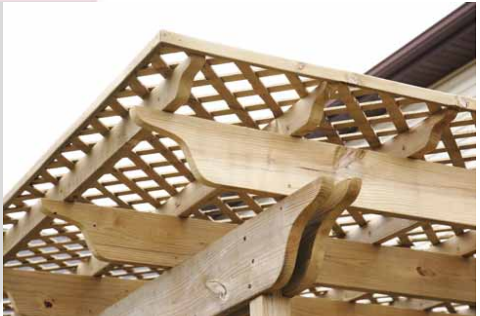
Above: A detail of the completed pergola shows the improved edge detail of the lattice, and the extra character created by spacing the main beams apart sandwiched over the 6x6 support post.
