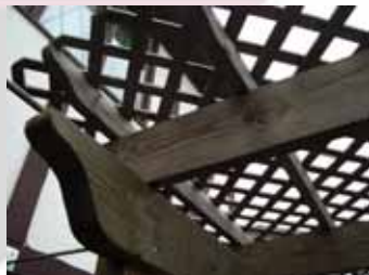
Left: The pergola was modeled after another pergola built years ago for another client of this Remodelor™. A handful of modifications and refinements were realized in the new version pictured above.
