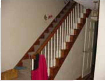
Before: the stairway railing was plain but extremely rickety.
